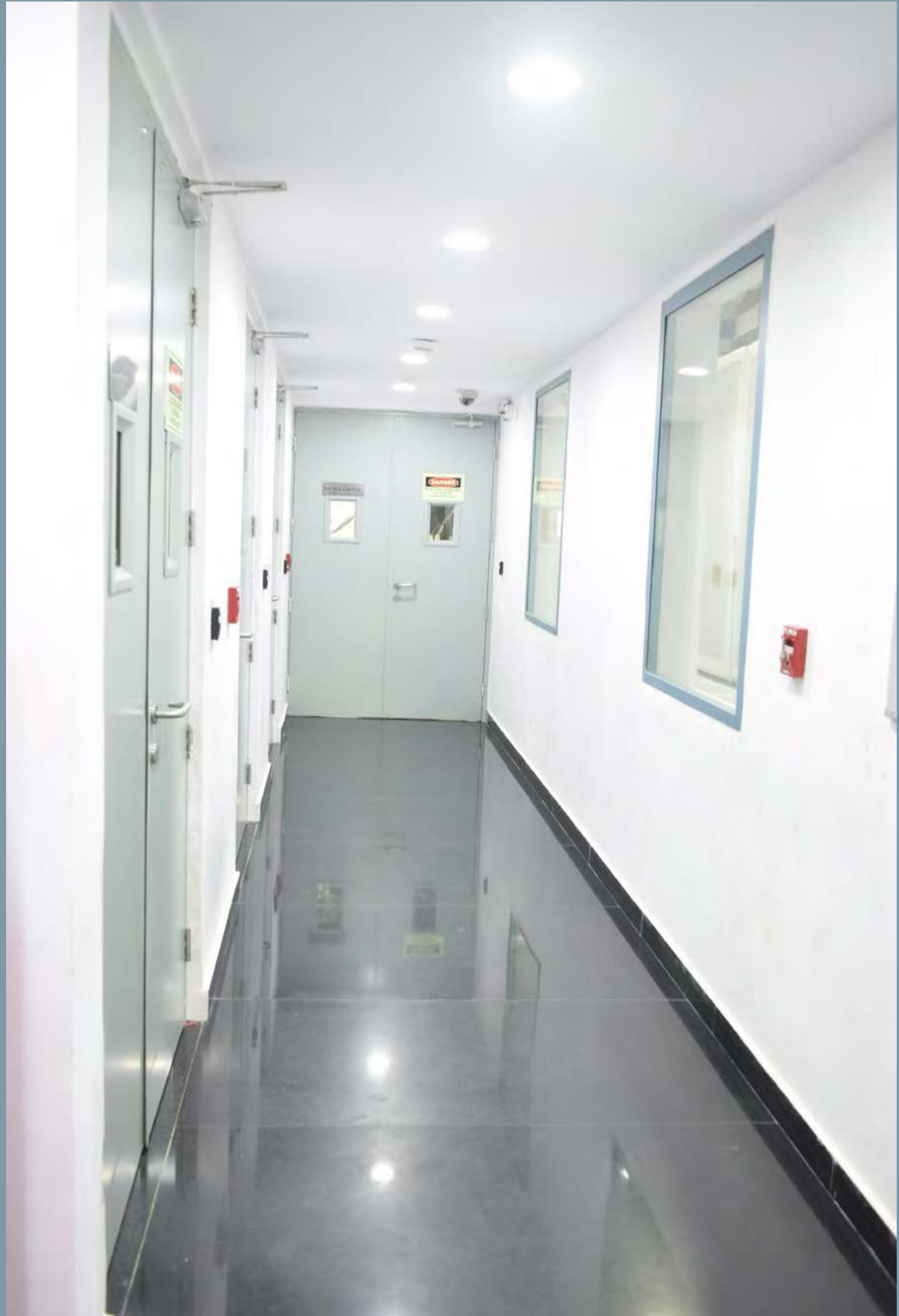
Data Center Corridor of Computer Services Centre
