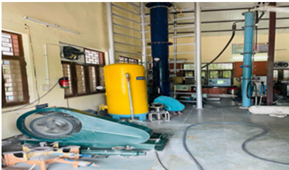
Biogas enrichment and bottling facility
